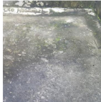
Leaking Overhead Tank
