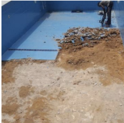
Leaking Swimming Pool
